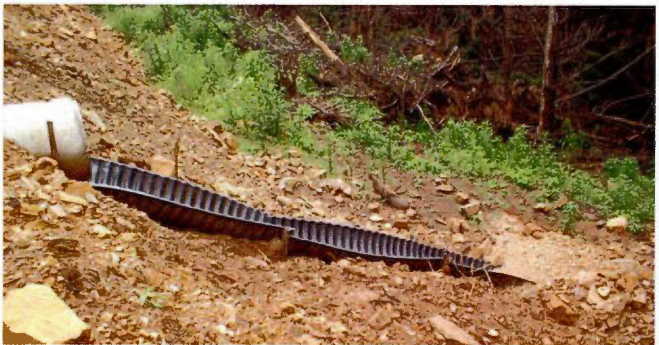
Figure 5.17: Drop-down structure and dissipater
