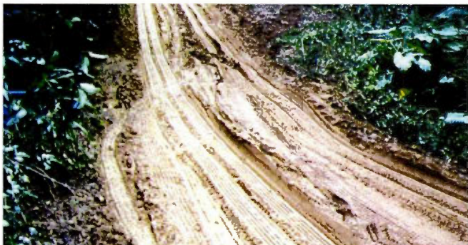
Figure 5.26: Example of road surface breakdown
