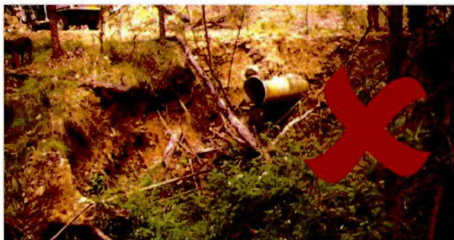
Figure 5.16: Example of poor outlet protection
