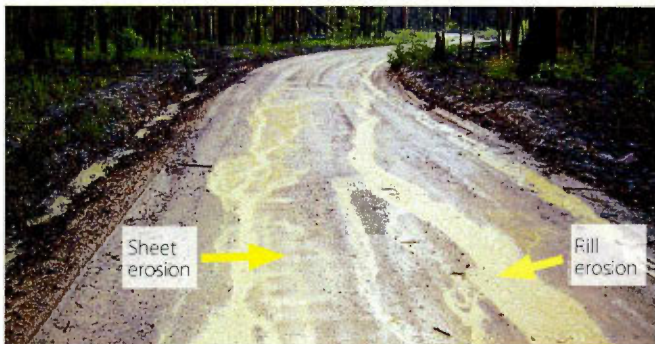
(a) Rill and sheet erosion
