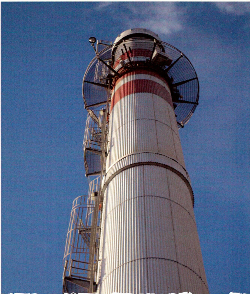
Monitoring stack emissions enables industry to prevent/minimise air pollution (DECCW)
