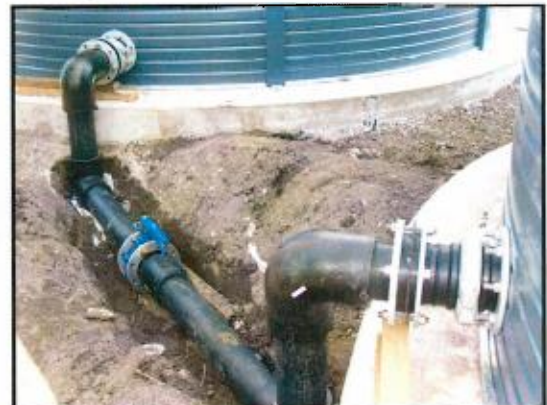
Figure 5: Balance pipe and control for Mackey Park tanks, December 2010.
