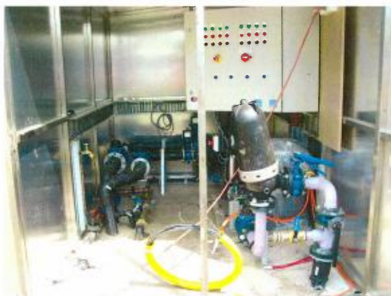
Figure 8: Mackey park pump house and irrigation controller, December 2010.
