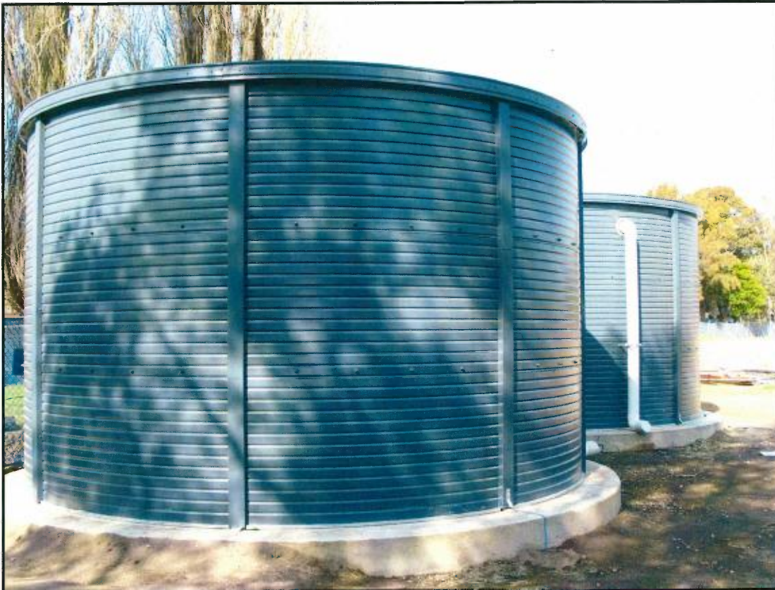
Figure 3: The two 75 kilolitre tanks at Mackey Park installed September 2010.
