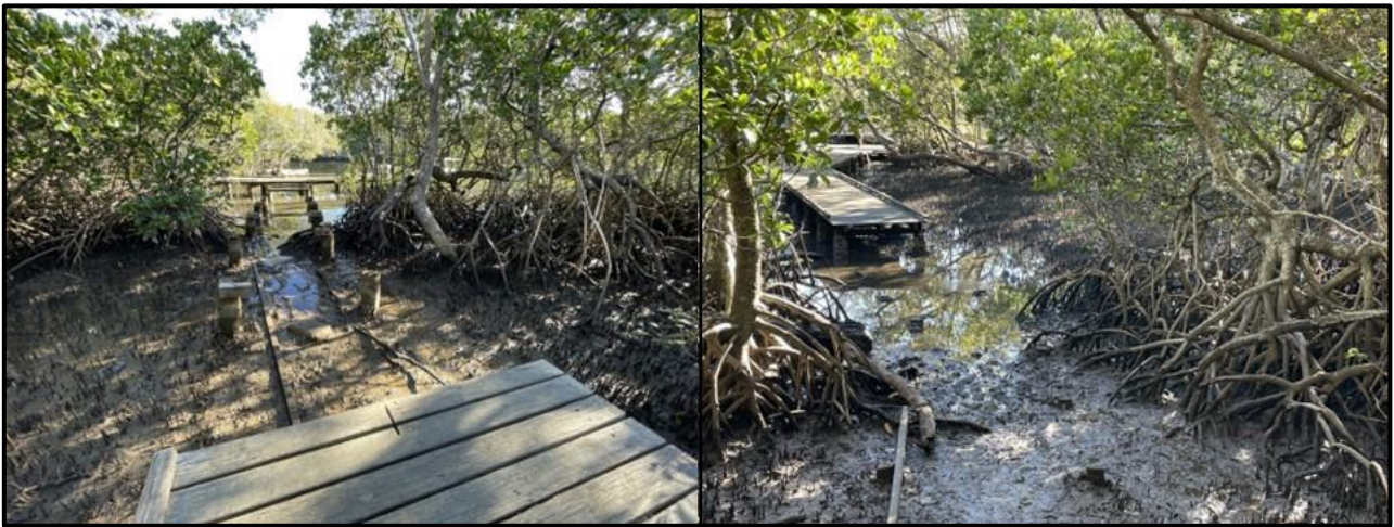
Figure 41 Damaged mangrove boardwalks at Ukerebagh Passage.
