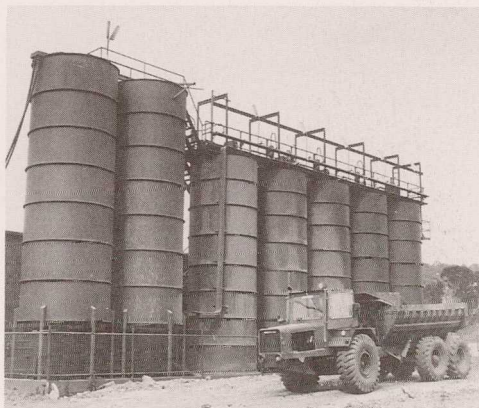
CIP plant, Browns Creek mine (Photo by Department of Minerals and Energy)
