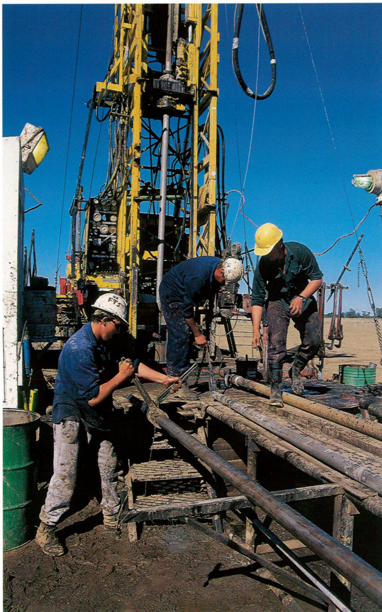
Drillers at work, exploring for gas at Coonarah near Narrabri in the Gunnedah Basin
