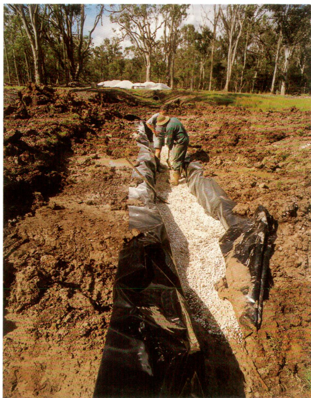
The anoxic limestone drain under construction at Glen Ayr. When sealed from the atmosphere, the limestone will neutralise the acidic water seeping from the old mine
