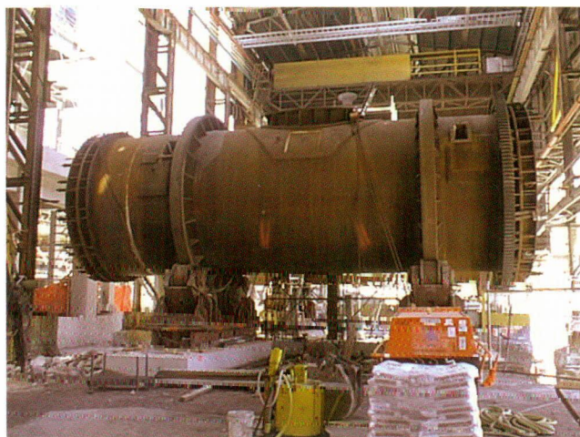
Anode furnace in place
