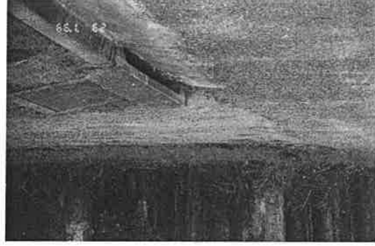
18. Tallong Rd – unsealed driveway, erosion
