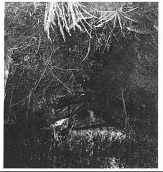
55. Stormwater outlet into river, Wauchope
