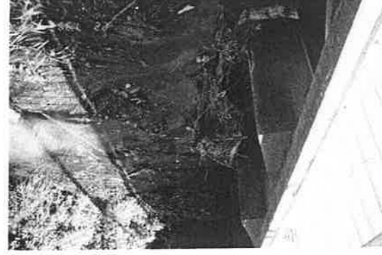
14. Algae, silt, litter and accumulation of tree branches in stormwater channel.
