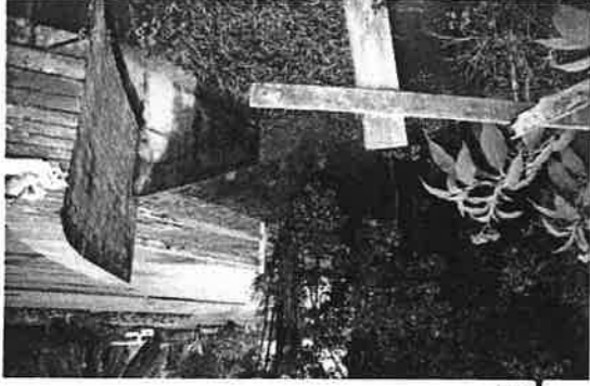
37. Stormwater channel – corner of Clareville Avenue and Bain Street – siltation, introduced species
