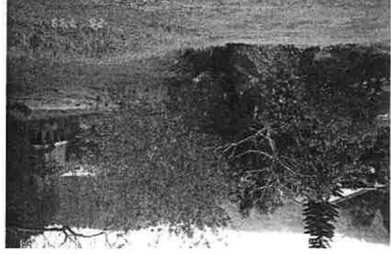
52. Stormwater channel – erosion, introduced species
