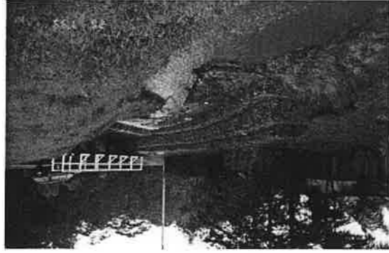
45. Stormwater channel with gabion to stabilise banks, a little bit of erosion where gabions end
