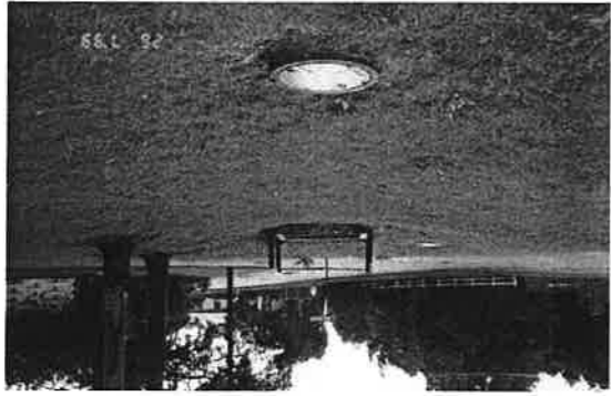
39. Grass swale leading into stormwater channel and runs through to where the above 2 photos were taken - accumulation of litter.
