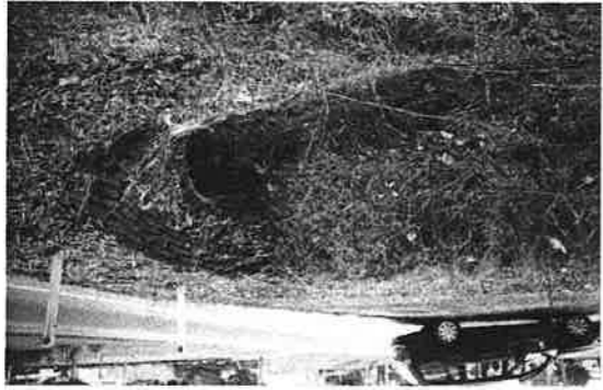
53. Siltation due to bank erosion, litter
