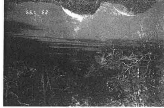
23. Bank erosion, Lakeside Woods Estate
