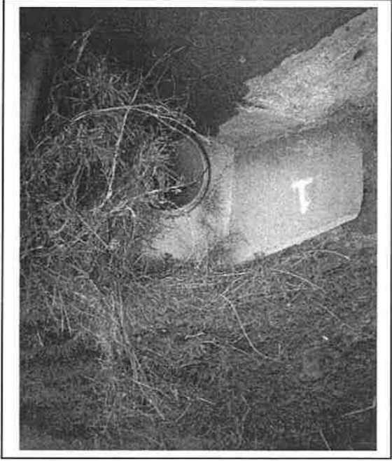
Stormwater outlet into Reserve, Wauchope (Note the pollution on this side of the Stormwater Channel)
