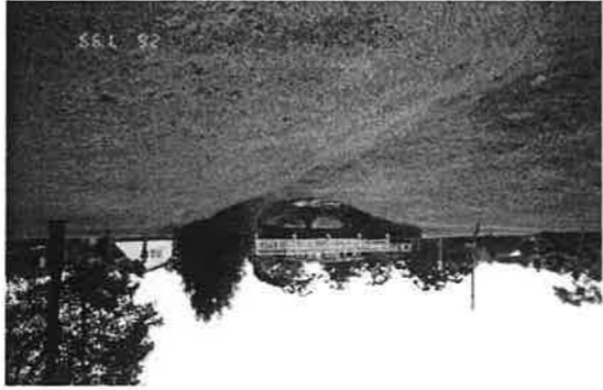
44. Same as previous but on the other side of the road, underground drain with grass swale on top
