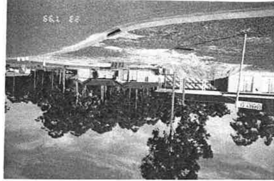
21. Stockpile with no silt fence, washing into stormwater pit
