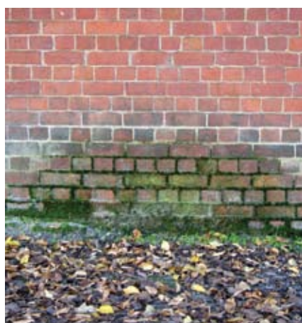
Figure 23 Maintenance, maintenance, maintenance. Here a roof gutter has rusted through and the colourful green damp zone is due to splash.
