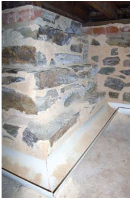
Figure 27 Semi-circular sections of PVC piping catch salt and other debris from sacrificial plasters and mortars on the walls beneath the floor of a church. Bedded on the same sacrificial mortar mix as that used for the walls, the pipes prevent the recirculation of the salts through the soils below and are cleaned out annually. White salts are visible on the stones in the centre of the photograph.
