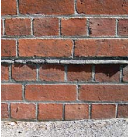
Figure 8 Many late nineteenth and early twentieth century DPCs were a mix of tar and sand that was laid hot. Being viscous, some have harmlessly extruded a little under the weight of the overlying masonry.
