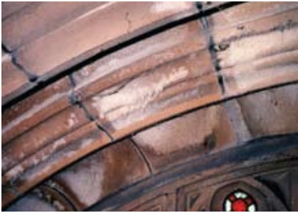
Figure 4 Thin needles of salt extruding from the top of a window arch. A slipped roofing slate punctured the copper roof gutter, allowing rainwater to wash salts into the stonework.
