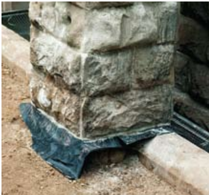
Figure 38 Insertion of a DPC by slot sawing. A mortar joint is sawn out with a chainsaw allowing insertion of DPC sheeting. As salt-laden stone is left above the DPC, the technique must be combined with desalination to be successful.
