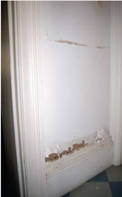
Figure 20 Evidence of previous treatment with hard impermeable plaster. Damp is evaporating from above and below the impermeable zone.
