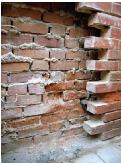
Figure 45 Decay of an inner leaf of brickwork into the cavity. This would not have been discovered had the wall not been opened up for undersetting of the outer leaf. The decay means that evaporation is occurring in the cavity in preference to the interior of the house. Multiple paint coatings or previous repairs of interior plasters with dense impermeable materials may be an explanation. Whatever the cause, the implications of decay occurring where it cannot be seen are profound. The inner leaf must be treated, using one of the methods described in this guide.
