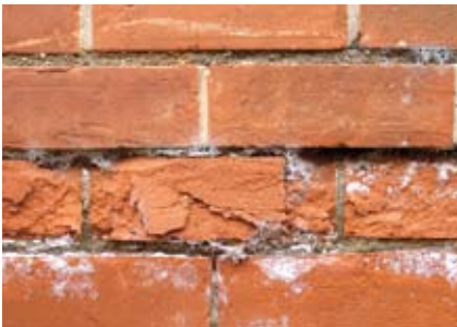
Figure 5 Salt attack in bricks causing disruption and loss of the fireskin, the harder outer surface that develops during firing in the brick kiln.
