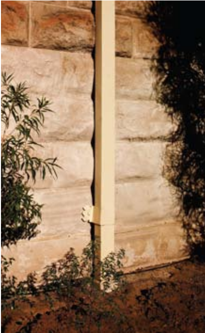
Figure 24 Garden beds against walls almost guarantee salt damp problems. Here the DPC was buried by 300 mm of soil — five courses of sandstone have been severely damaged.
