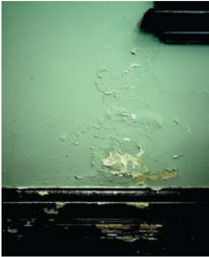
Figure 7 Typical blistering of paintwork and damage to internal plaster due to the combined effects of rising damp and salt attack. The skirting is a cement moulding and also shows salt damage.
