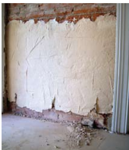
Figure 32 Absorbent poultice shortly after application to an interior wall from which plaster has been removed. The poultice is left on the wall until it is dry, which may take 2–3 weeks depending on weather conditions.
