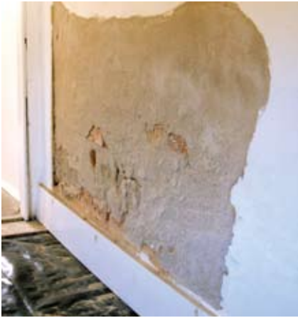
Figure 31 Sacrificial plaster decaying as intended. Plastic sheeting is used to catch the salts and prevent their recycling through the soils and walls.
