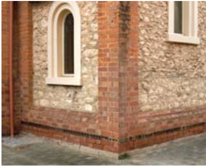
Figure 37 Undersetting from the 1930s. New bricks and stones have been inserted up to a line above the window sill on the left. Bricks below the DPC are visibly damp (see also Figure 10).
