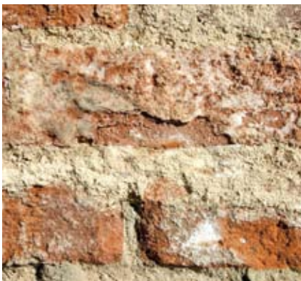
Figure 52 A thick film of salt that crystallised beneath a hard render, which was in turn finished with a high-build (thick) paint coating. For evaporation (and hence salt crystallisation) to occur the render must first have become partially detached from the brickwork. Thermal cycling would then drive air movement, allowing evaporation. The salt was chiselled off and the brickwork poulticed before re-rendering.
