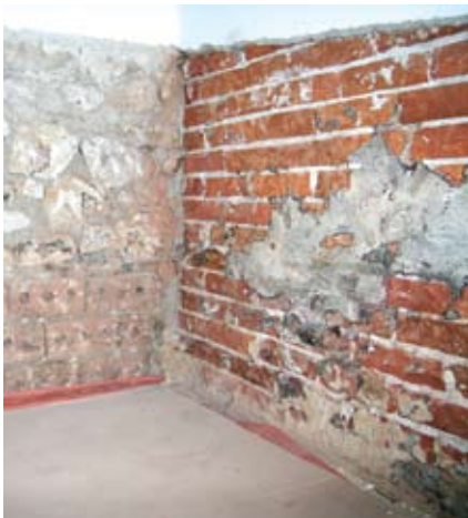
Figure 51 Discoveries on removing plaster from interior walls. On the left, the brick-on-edge is a partial undersetting of the inner part of a solid wall, leaving the outer part untreated — a total waste of effort. On both walls, but more apparent on the right, are remnants of a dense hard cementitious material containing milled iron that was designed to rust and block pores, making it impermeable. Its removal proved extremely difficult.
