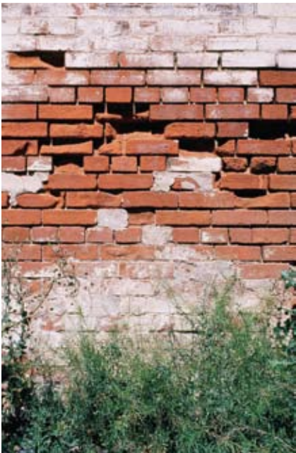
Figure 2 Typical salt damp damage in Adelaide, with decay of the bricks extending from about 0.5 to 1.2 metres above ground. There are no obvious signs of salt because it has been washed off by rain. Paler (underfired) bricks are more susceptible to salt attack than the darker, more well-fired ones.
