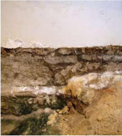
Figure 53 Damaged plaster on a damp wall; the dampness is indicated by green algae and white salts crystallising on the stonework and fill below. The recent plaster is decaying because it contains gypsum.
