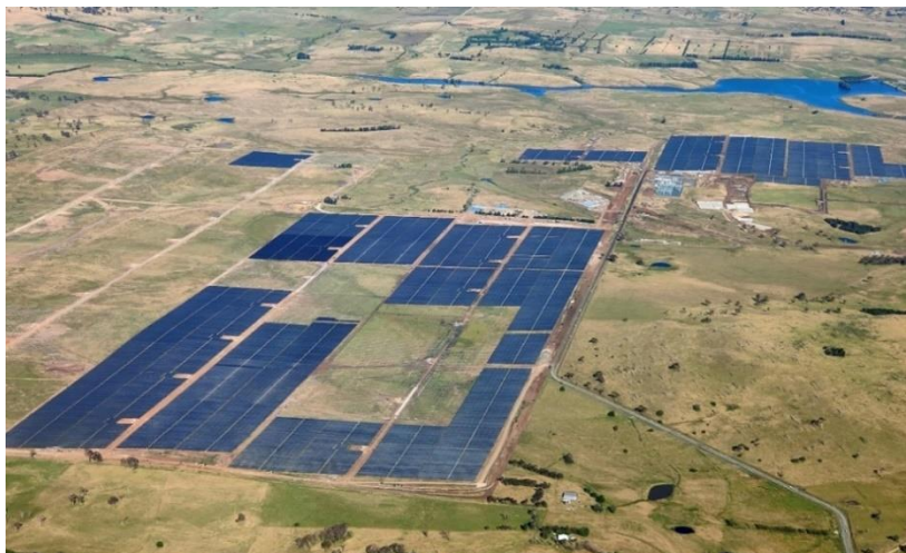
Figure 18: New England Solar Farm under construction near Uralla. Photo credit: Matthew Smith.
