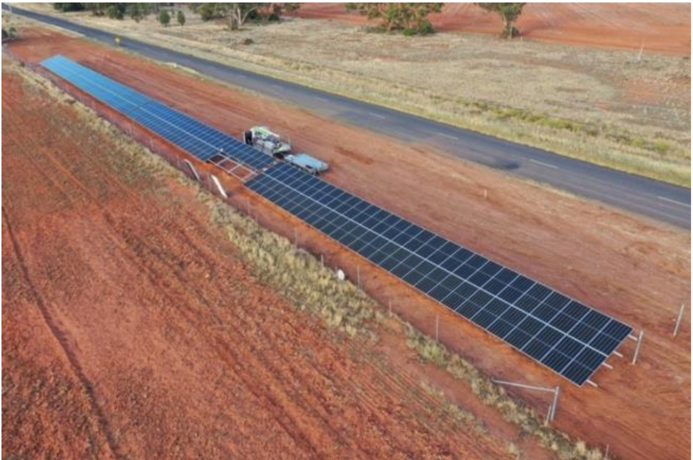
Figure 8: Solar panels in the Lachlan shire. Photo credit: Lachlan Shire Council.
